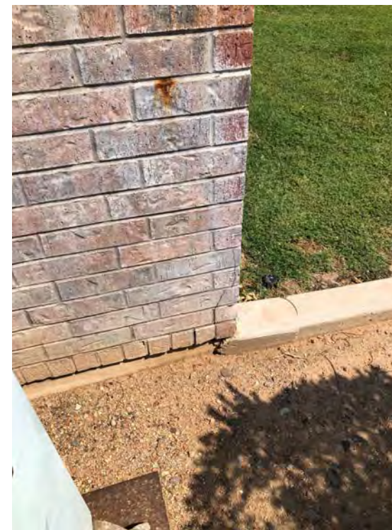
Brick Cracking at Outdoor Classroom
