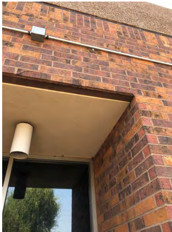
Brick Cracking Possibly Caused by Steel Lintel Corrosion
