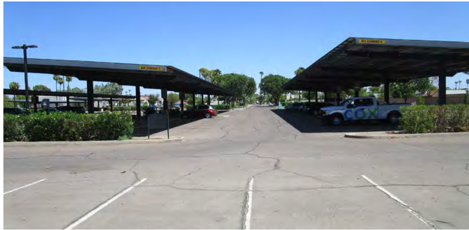
Solar shade canopies at South parking area
