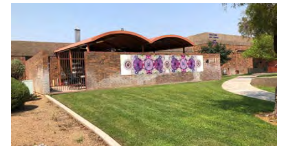
Water Stains on Brick at Outdoor Classroom
