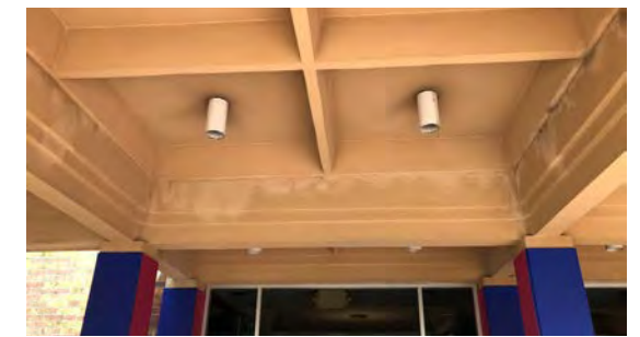
Water Stains at Entry Canopy
