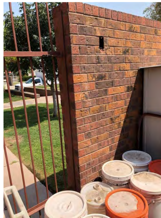
Brick Cracking at Outdoor Classroom
